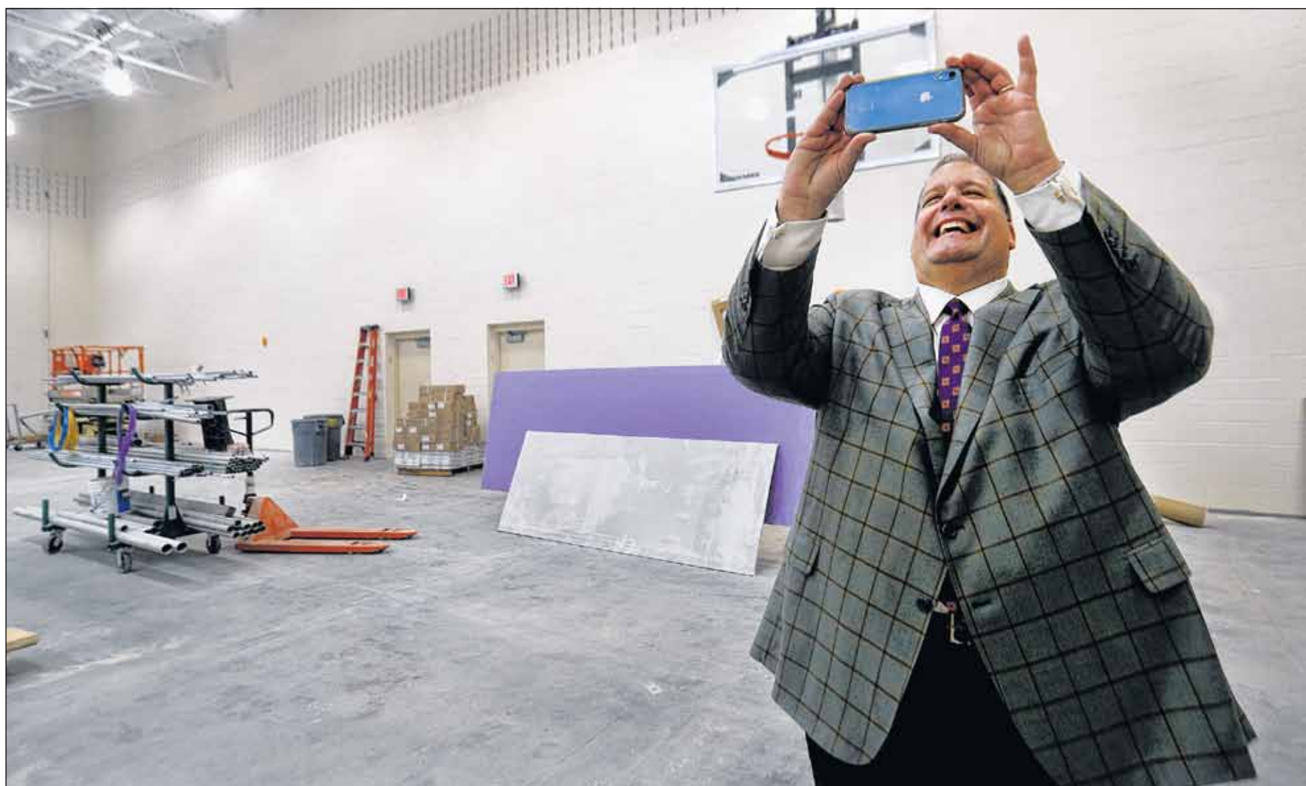
David Schwager take a photo of the progress on the new gymnasium in the Jewish Community Center in Kingston.
